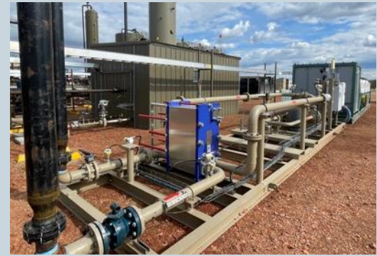
Fluid Cooling Williston Basin, ND
